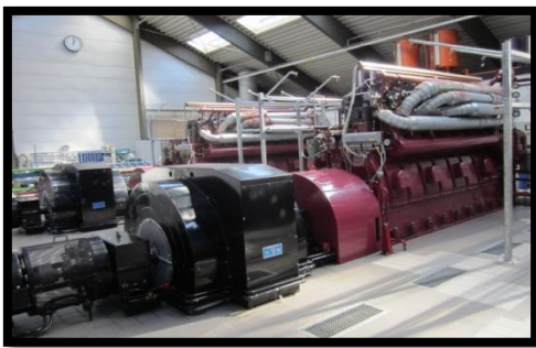
Figure 178 - The generators in Narsaq
