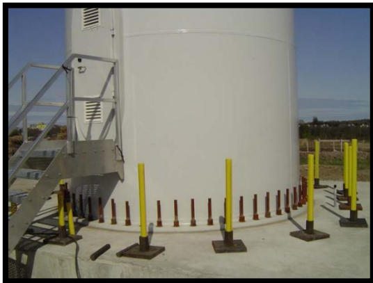
Figure 149 - Bottom of turbine tower is mounted on concrete plate area (Earth Systems)
