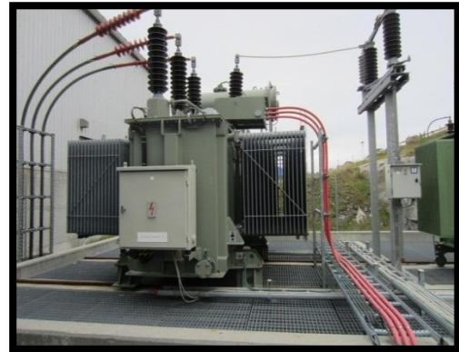
Figure 183 - HV transformer outside of the switch-gear facility, Nukissiorfiit Qaqortoq.
