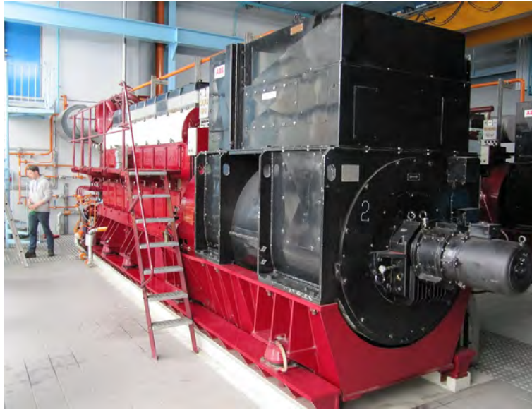
Figure 18: One of the two main diesel generators.
