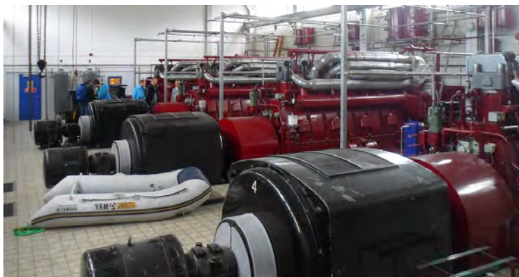
Figure 19: Three of the four backup diesel generators.
