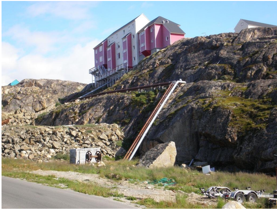
FIGURE 9: OVERGROUND DISTRICT HEATING PIPES BETWEEN VV3 AND VV4, IN AUGUST 2011.
