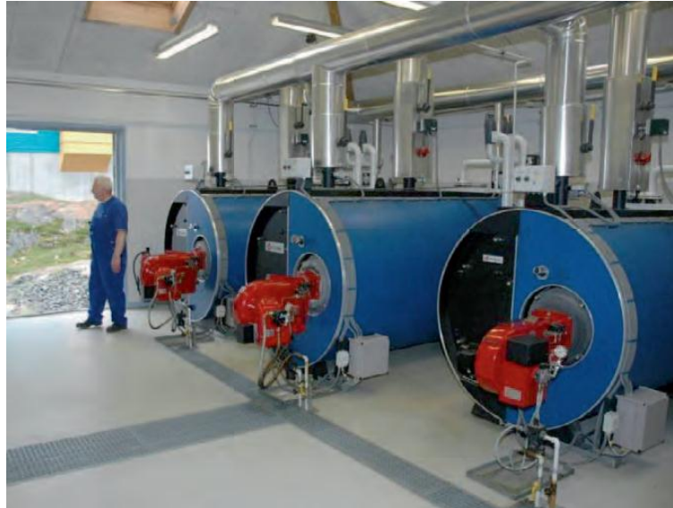
FIGURE 12: OIL BOILERS IN DISTRICT HEAT PLANT VV3 (16)
