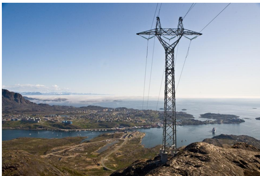
FIGURE 7: THE ELECTRICITY SUPPLY LINE LINKING THE HYDROPOWER PLANT TO SISIMIUT (14)
