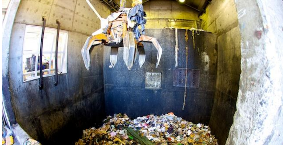
FIGURE 17: WASTE PIT AND GRAB SEEN FROM THE RAMP AREA IN SISIMIUT. THE WASTE FUNNEL IS BEHIND THE BACK WALL (12).
