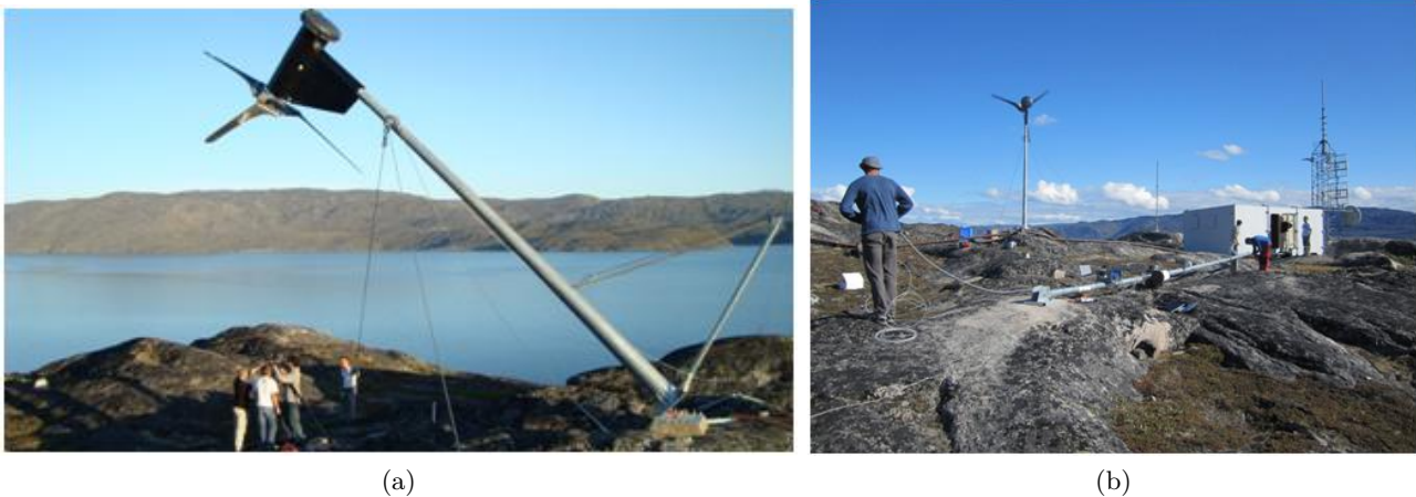
Figure 37: Works on existing turbine and met. mast. (a) process of pulling down the turbine and placing the tripod at the right position (b) Working on the existing mast
