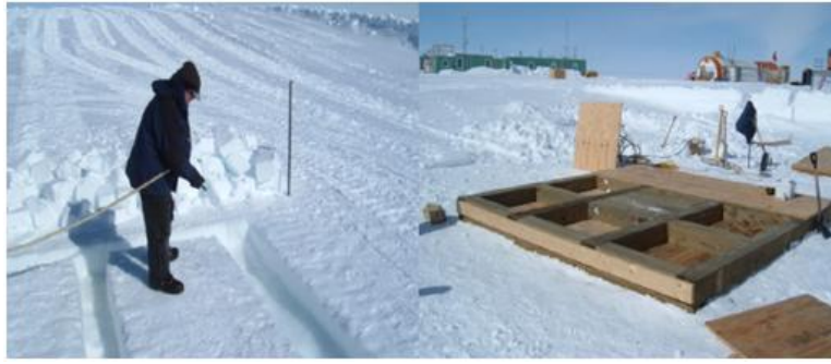
Figure 16: foundation strategie for the Proven Wind Turbine at the Summit Station, Greenland.
