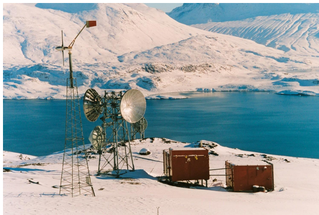
Figure 58: TG's first venture in a wind turbine; picture provided by TELE Greenland A/S.
