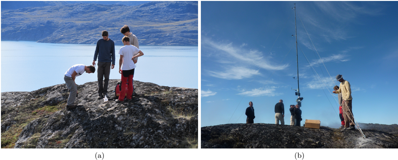
Figure 44: New met. mast erection process. (a) Drilling the holes to anchor the guy wires of the new met mast (b) New met mast erected at Sarfannguaq
