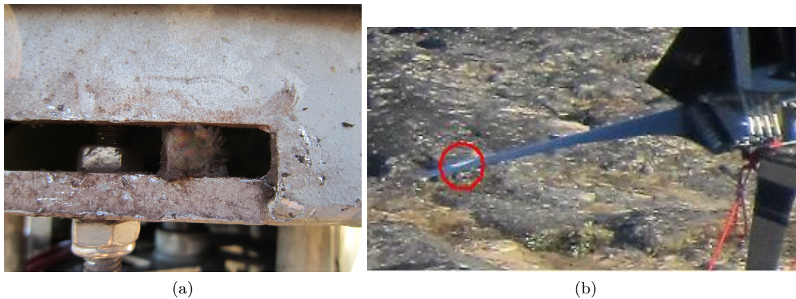
Figure 40: Maintenance work on the turbine. (a) Lump of magnet from the generator (b) Patch applied on the cracked blade
