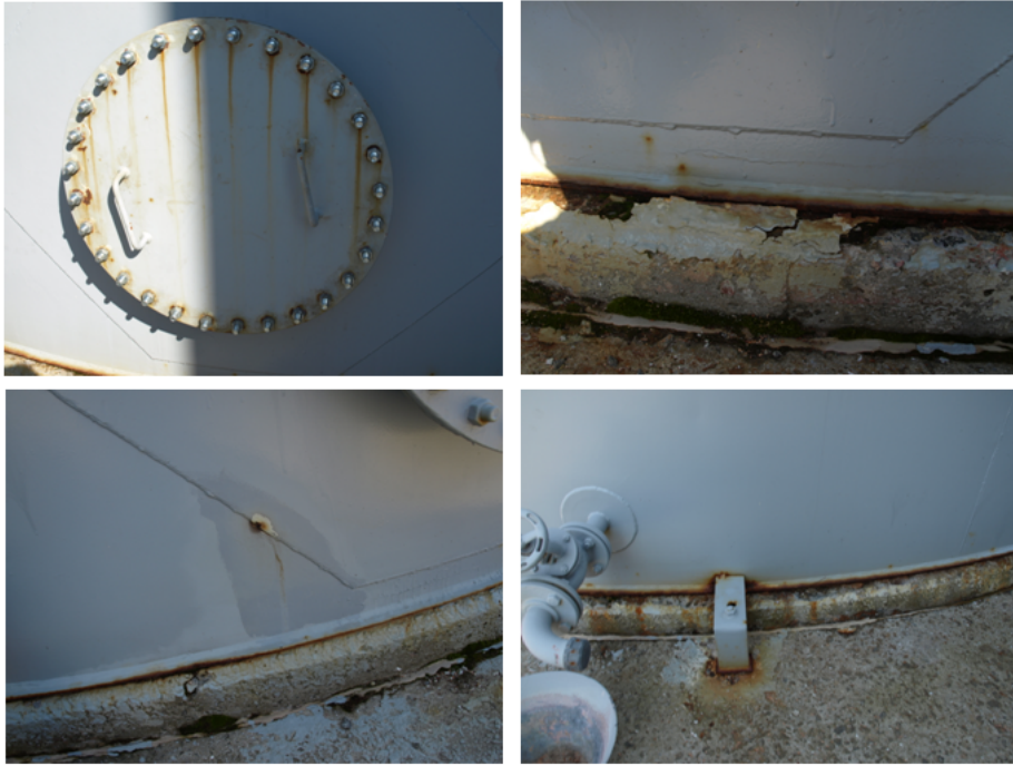
Figure 6: Corrosion on the tanks
