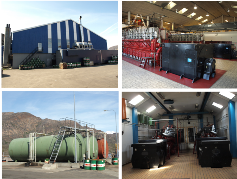
Figure 25: Facilities of power plant
